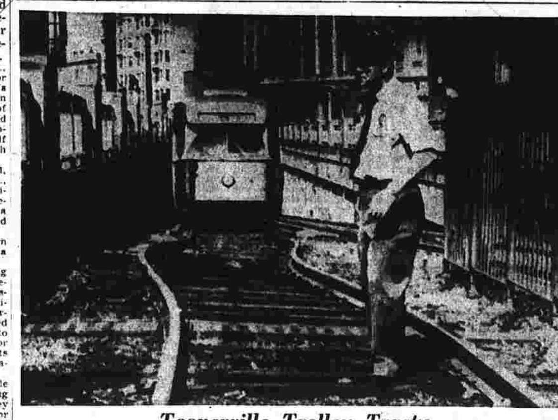
When the heat hit 95 yesterday in Boston—highest mark of the year—it was what happened to MTA tracks at Huntington Ave. Despite the heat-warped rails, cars were able to move slowly over the roller-coaster section. (AP Photofax).
